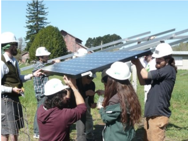
Blue Lake Rancheria: Volunteers install residential solar in the community (March, 2015) Photo Credit: GRID Alternatives
